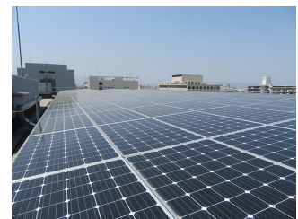
Solar power panels on a rooftop of the Kashima Site office building
